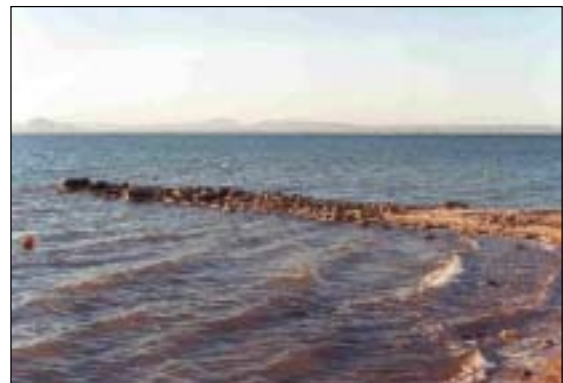
Fig. 33: Groin construction to stop sand losses in the Mar Menor shore of La Manga.
